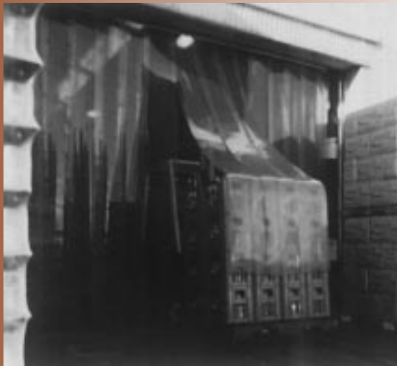
Clear vinyl strip installed on loading dock door allows easy access while offering thermal protection and noise reduction.
